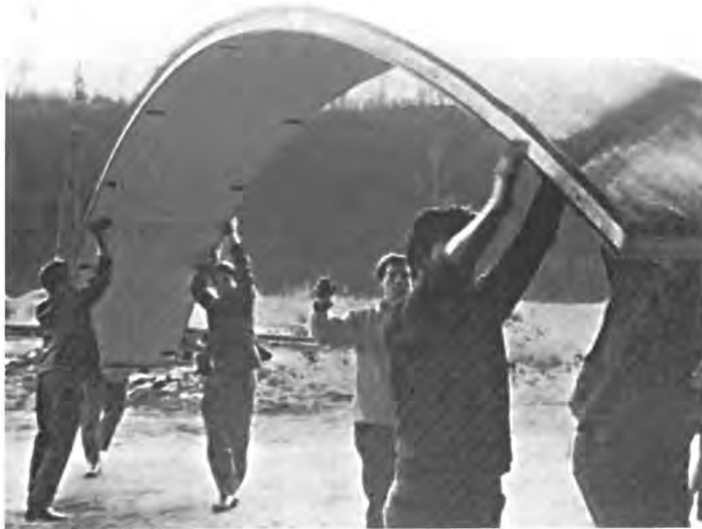
Figure 16. Youth Club, Ermont (Val d'Oise), 1966. Building under construction. (© Centre Pompidou, Bibliothèque Kandinsky)
