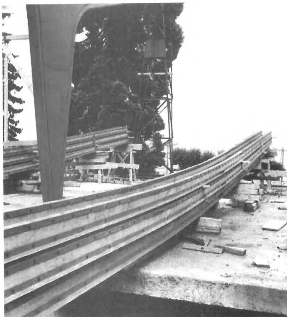
Figure 13. Pump Room, Evian (Haute-Savoie), 1956. Building under construction showing curved roof beam. (© Centre Pompidou, Bibliothèque Kandinsky)
